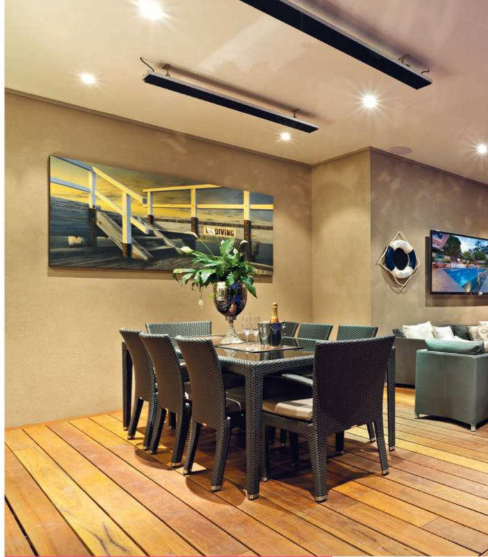
Electric strip heaters mounted in this outdoor zone make a great room comfortable all year round.
